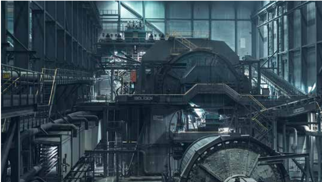
◀ The mill in the concentrator at Aitik.
